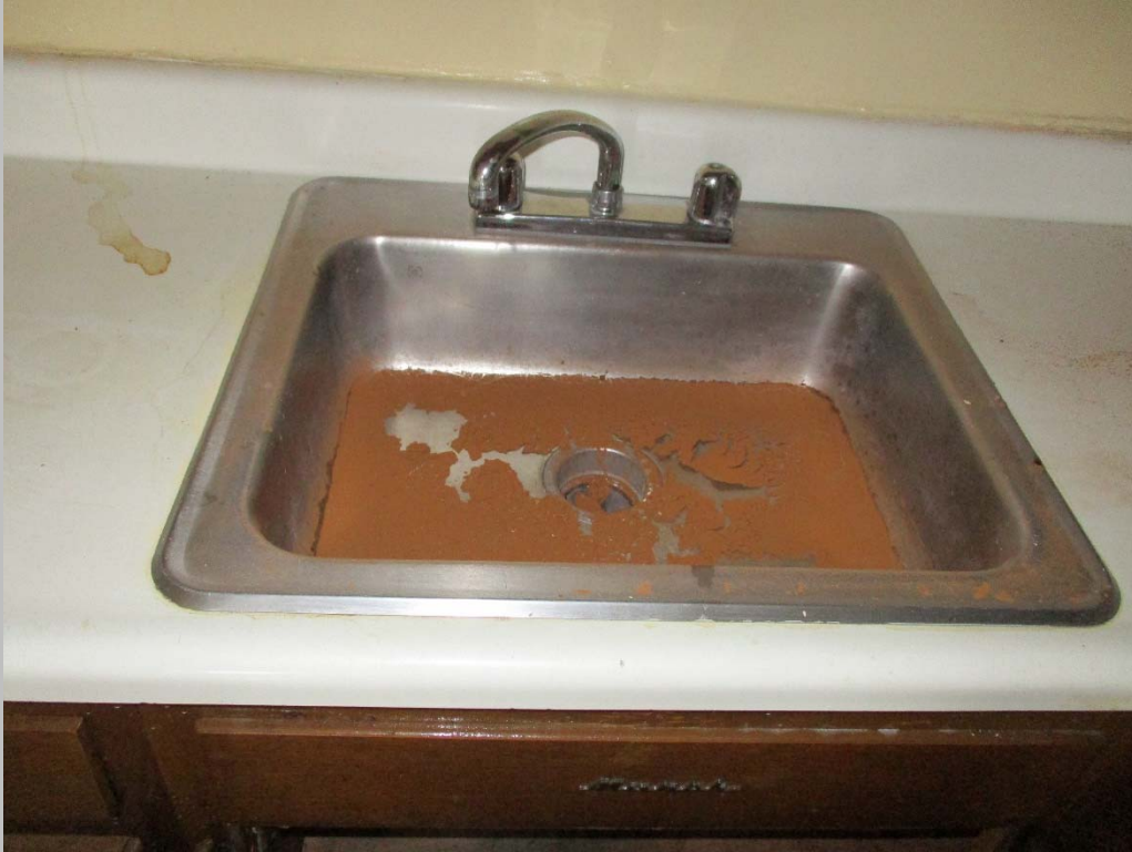
Dwelling unit sinks experience frequent backups throughout
