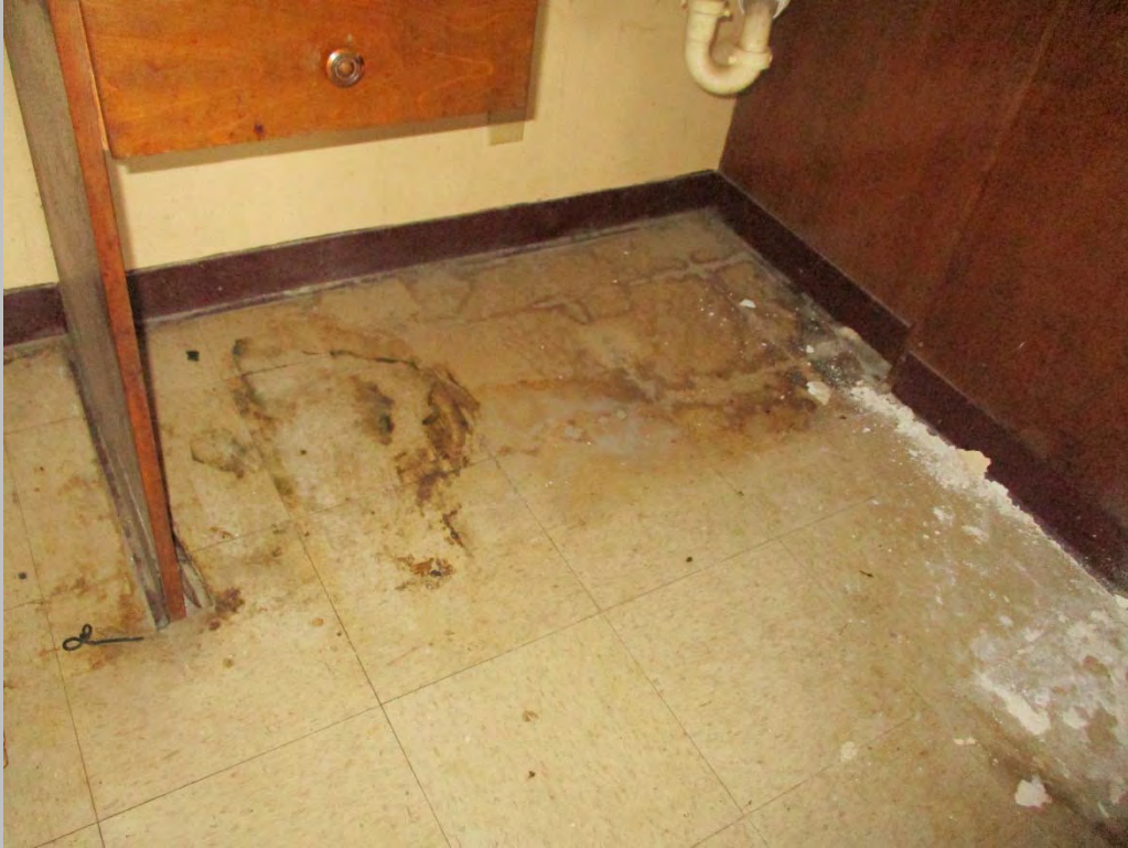
Water damaged VCT flooring throughout
