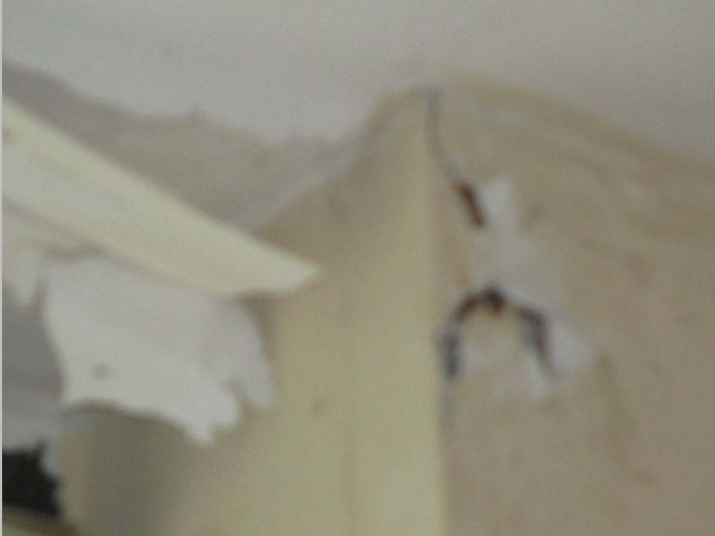
Water damaged ceilings throughout
