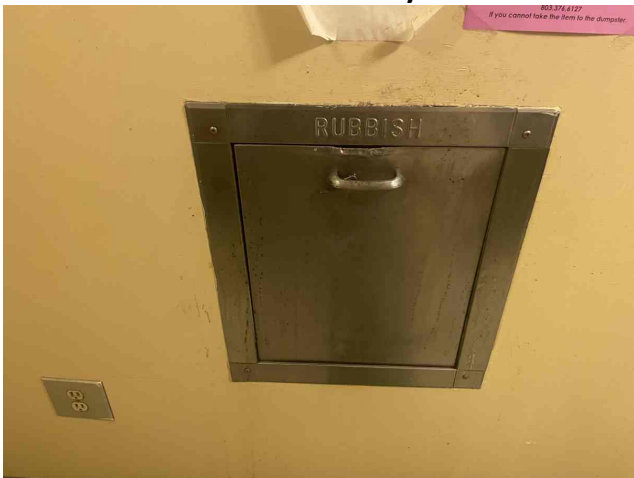
Central Trash System
