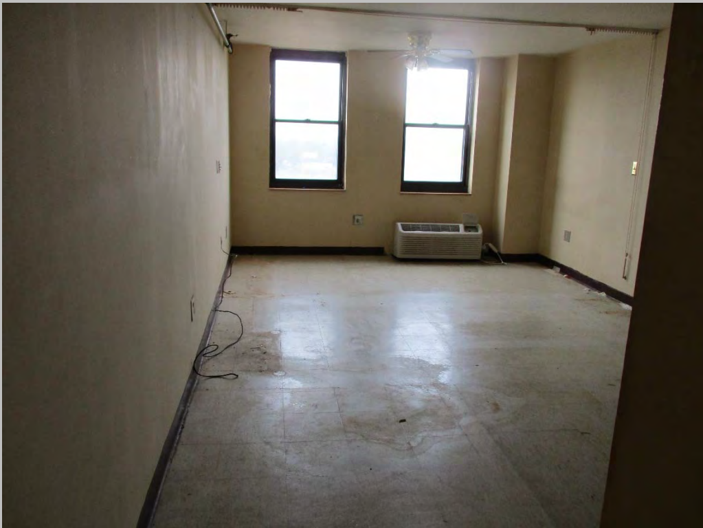
Water damaged VCT flooring throughout
