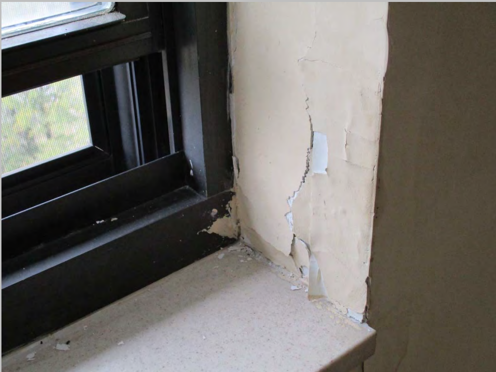
Wall damage due to exterior water infiltration throughout
