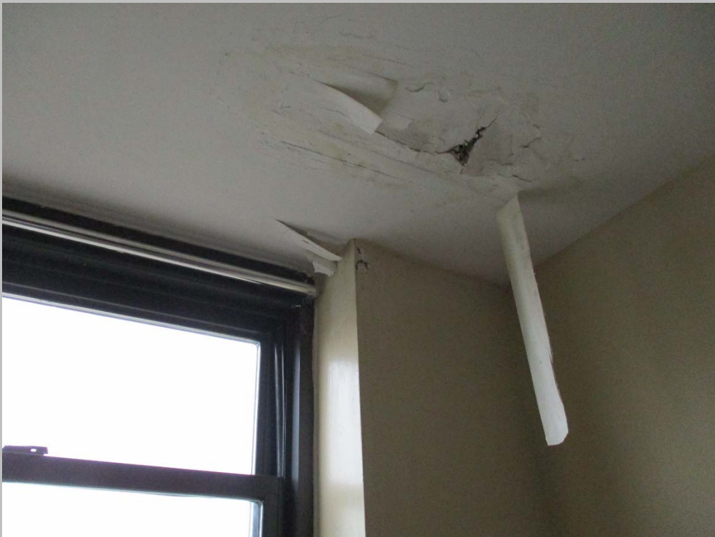
Water damaged ceilings throughout
