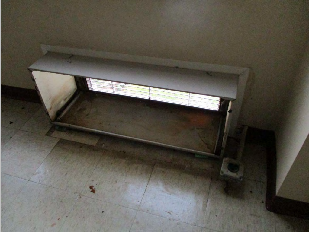
Flooring damage due to exterior water infiltration throughout
