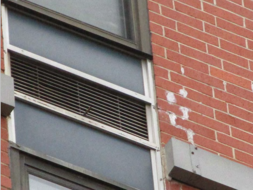
Significant cracking of the brick façade throughout
