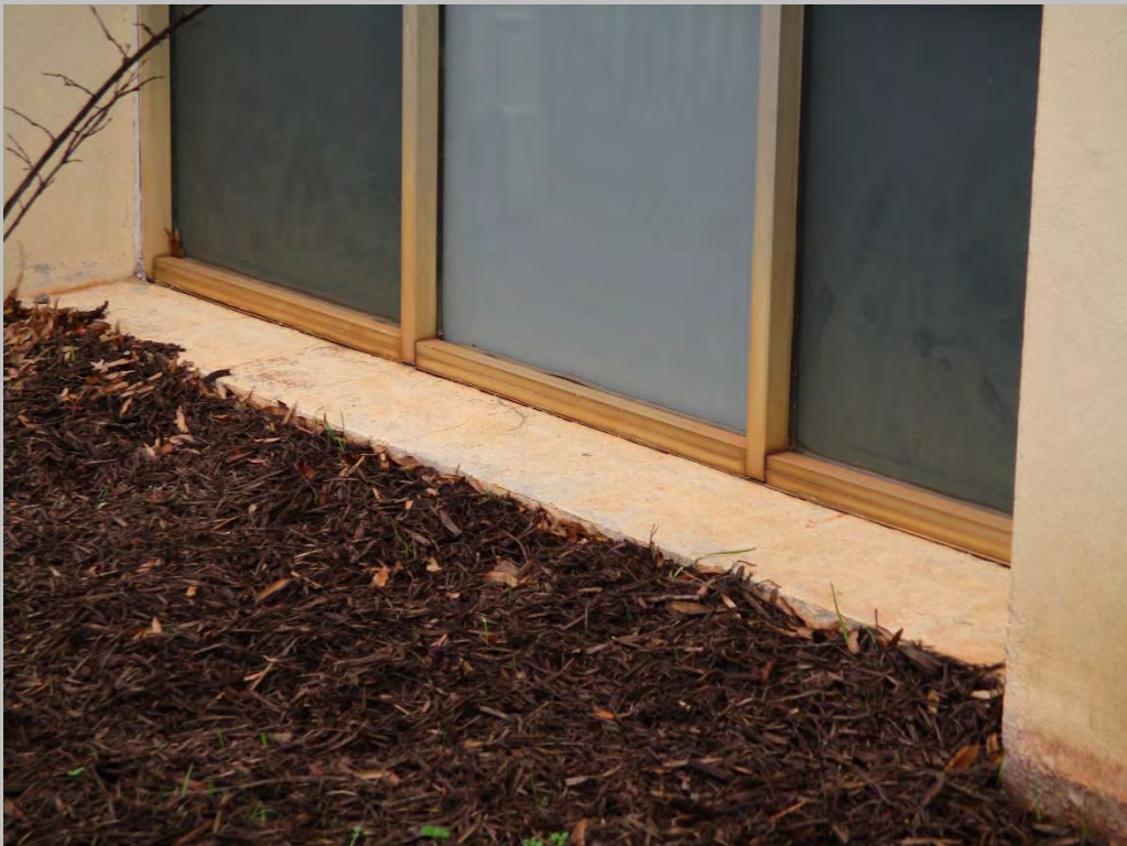
Failing sealants at all glass storefront window assemblies
