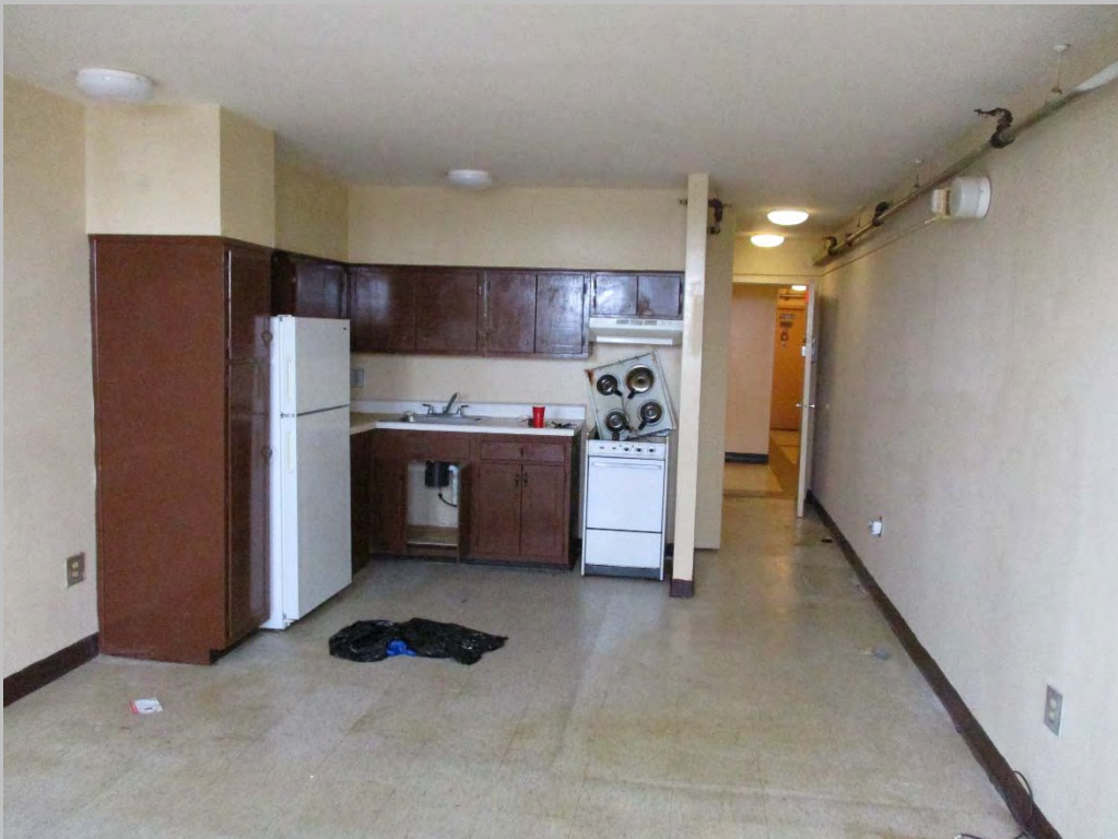
Water damaged VCT flooring throughout
