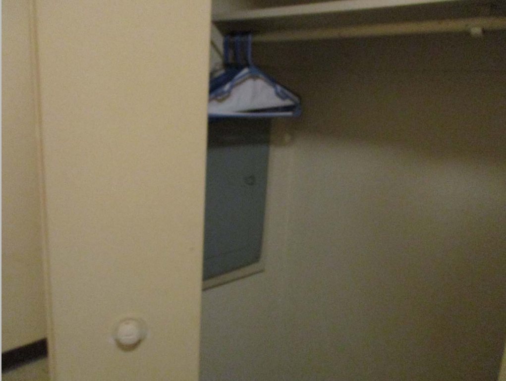
Electrical panels installed in closets throughout
