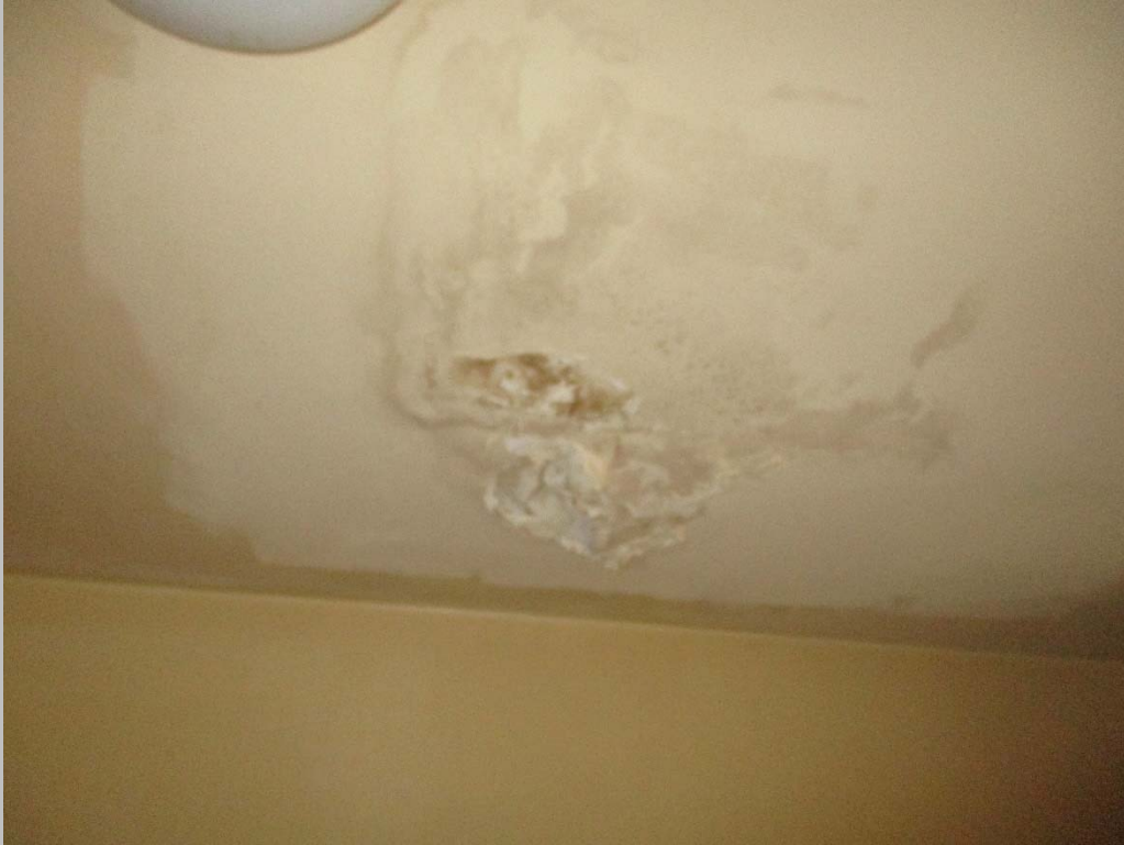
Water damaged ceilings throughout
