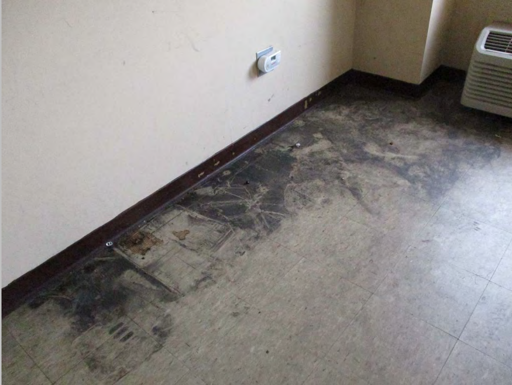
Water damaged VCT flooring throughout
