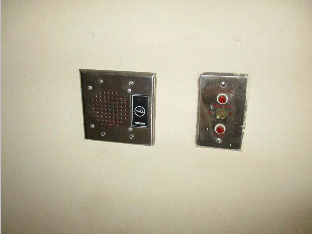
Typical non-compliant emergency call unit
