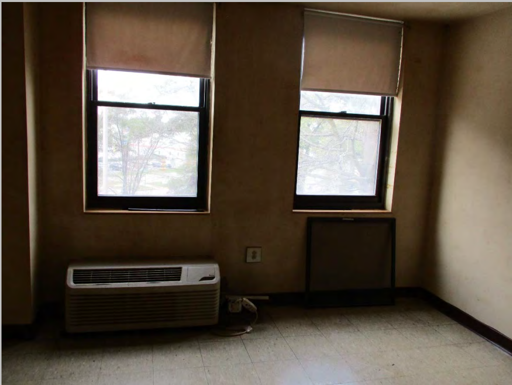
Water damaged VCT flooring throughout
