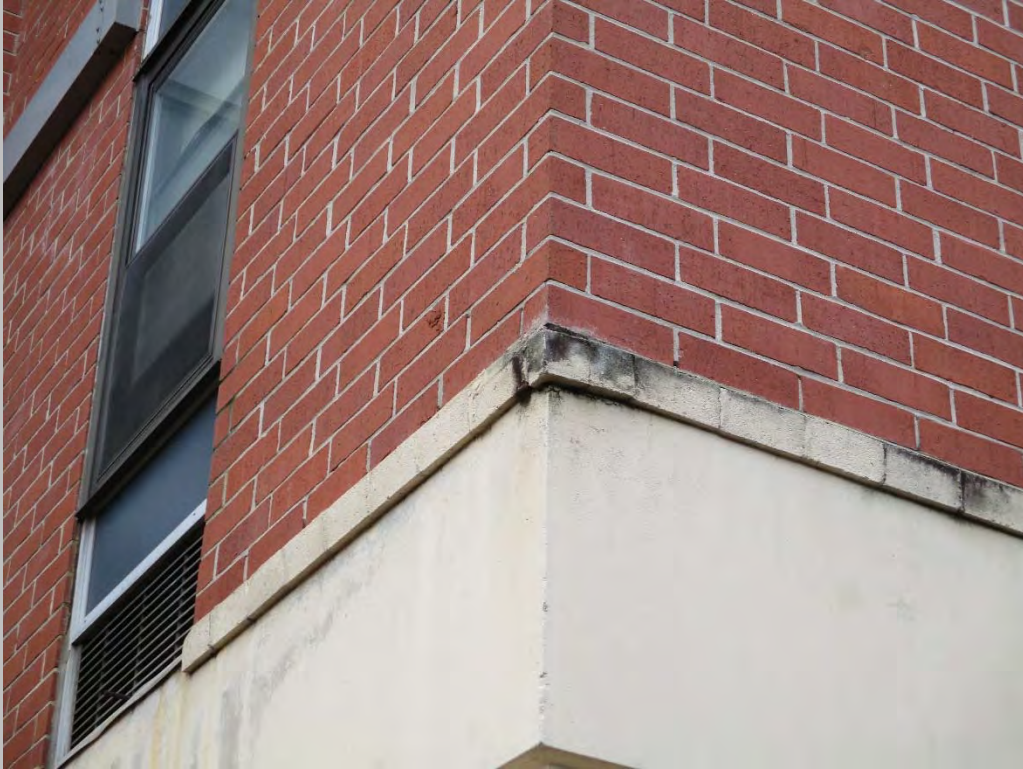
Significant cracking of the brick façade throughout
