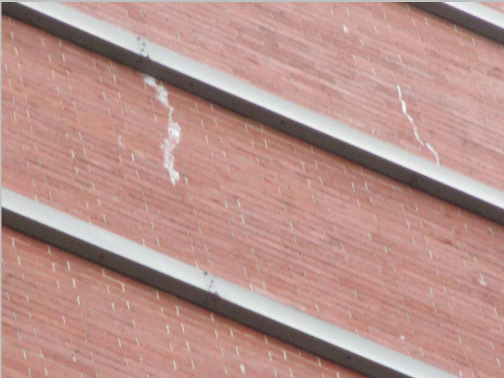
Significant cracking of the brick façade throughout
