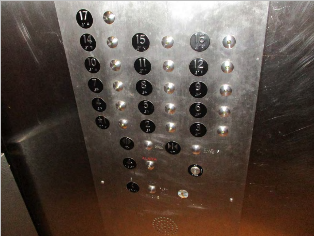
Typical elevator control panel
