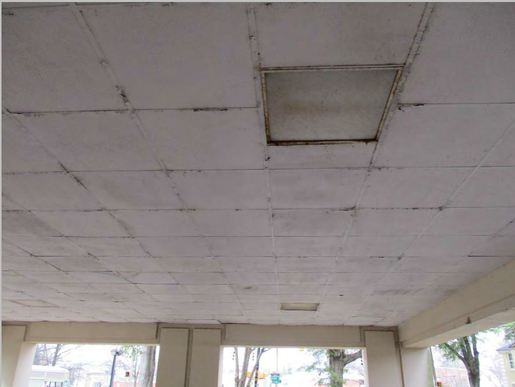
Porte cochere ceiling in poor condition
