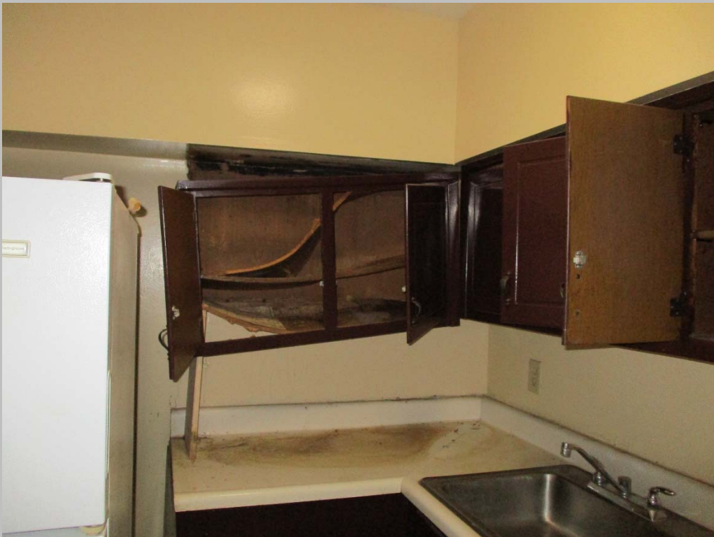
Typical dwelling unit kitchen cabinetry with water damage
