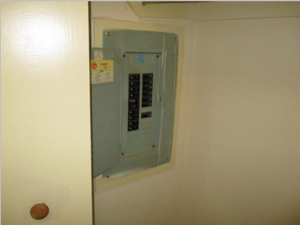
Electrical panels installed in closets throughout
